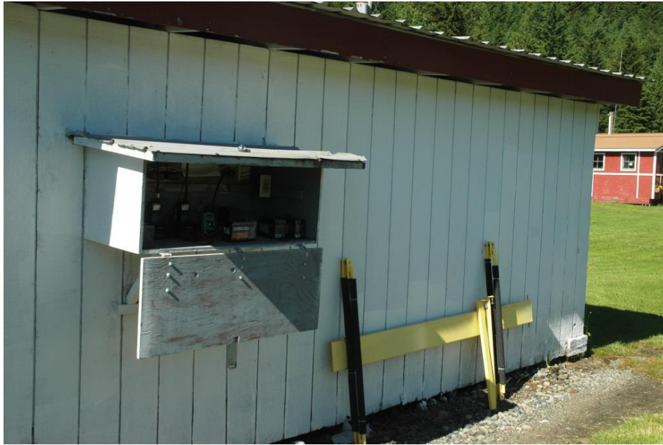
Figure 15 Battery Charging Station Outside of Shed
