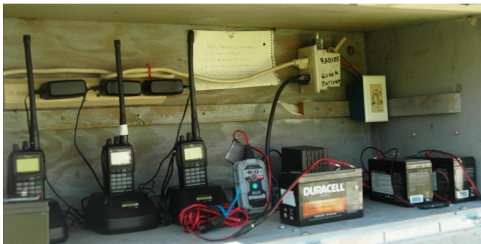
Figure 16 Inside of Battery Charging Station
